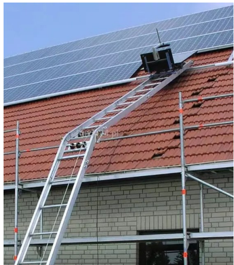
• Solar Panel Roof
